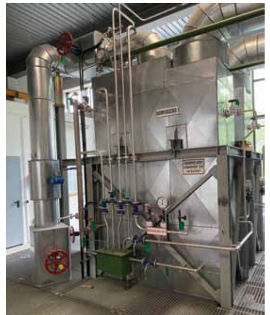
➤ Old heating condensers with 2 x 18 MW.
